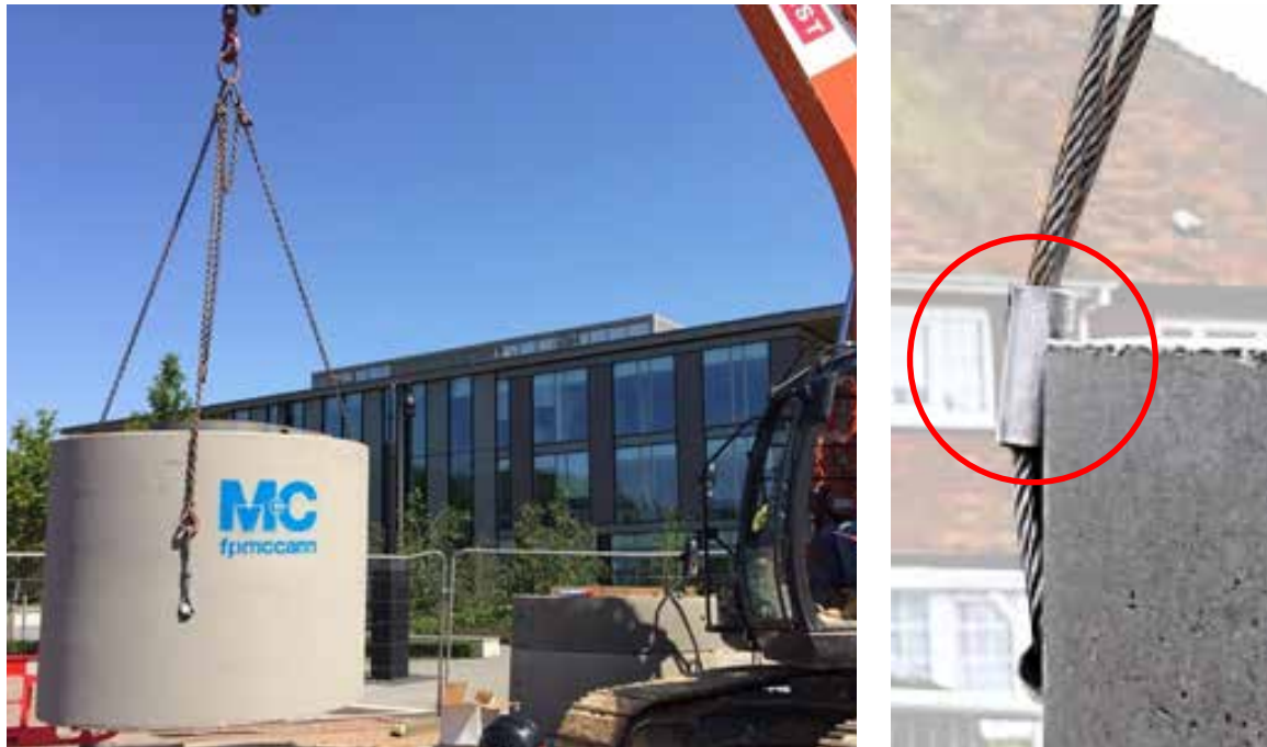
Figure 9 - Site image: Main unit lifted using provided spherical anchors, with edge protection (right)
