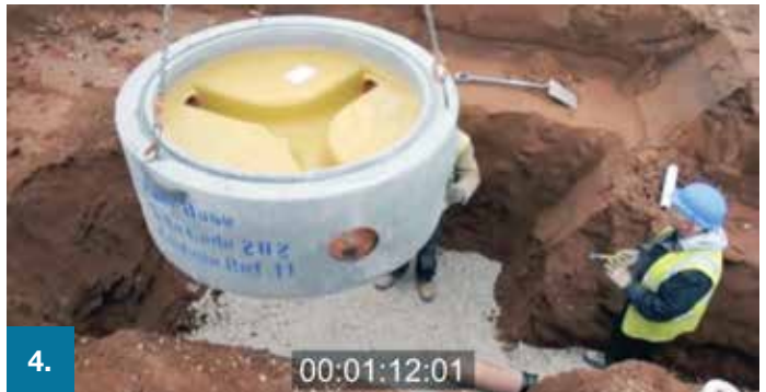
4. The easi-base unit is safely lifted and lowered into place using 3 integral lifting loops.
