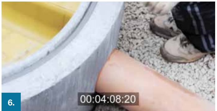
6. The easi-base unit is set level, a gradient of 1:10 is present at the benching with a run-off towards the outlet.
